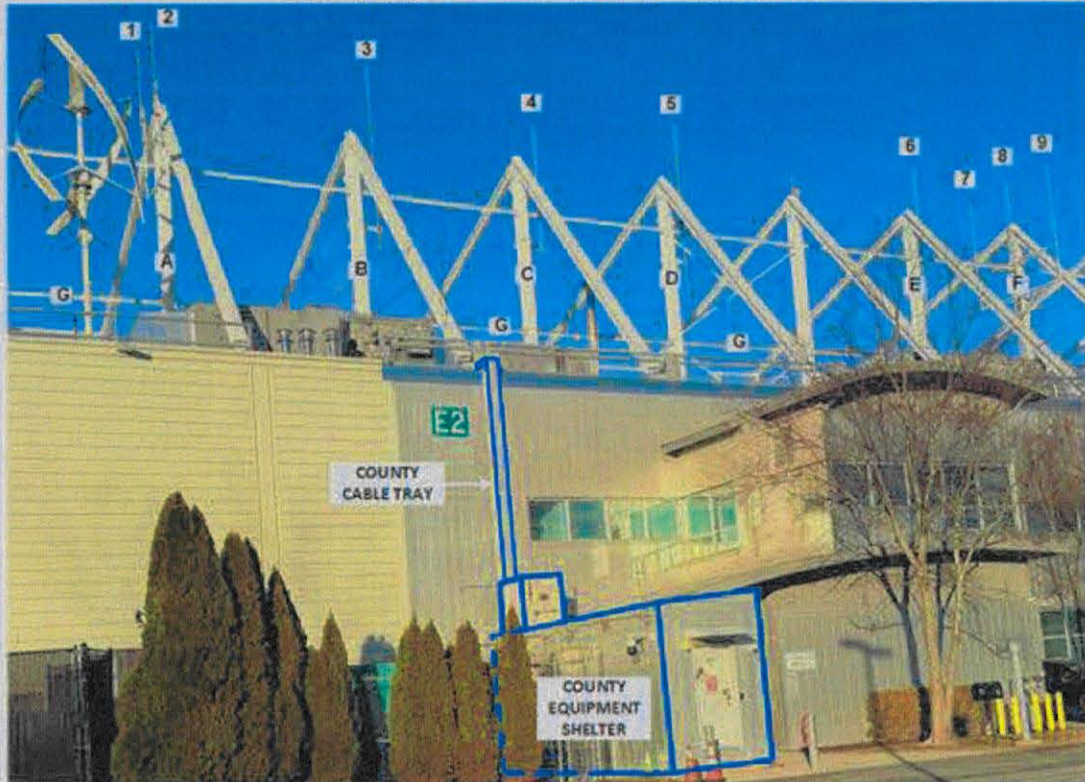
County Antenna Masts are numbered '1' through '9'. County transmission lines to be routed inside County Cable Tray from County Equipment Shelter to steel column 'C' on roof, clamped along lateral steel bracing 'G' to steel columns 'A', 'B', 'D', 'E', and 'F'; and up steel columns 'A' through 'F' to County Antenna Masts '1' through '9'. Existing County Antenna types are described on the following pages.
